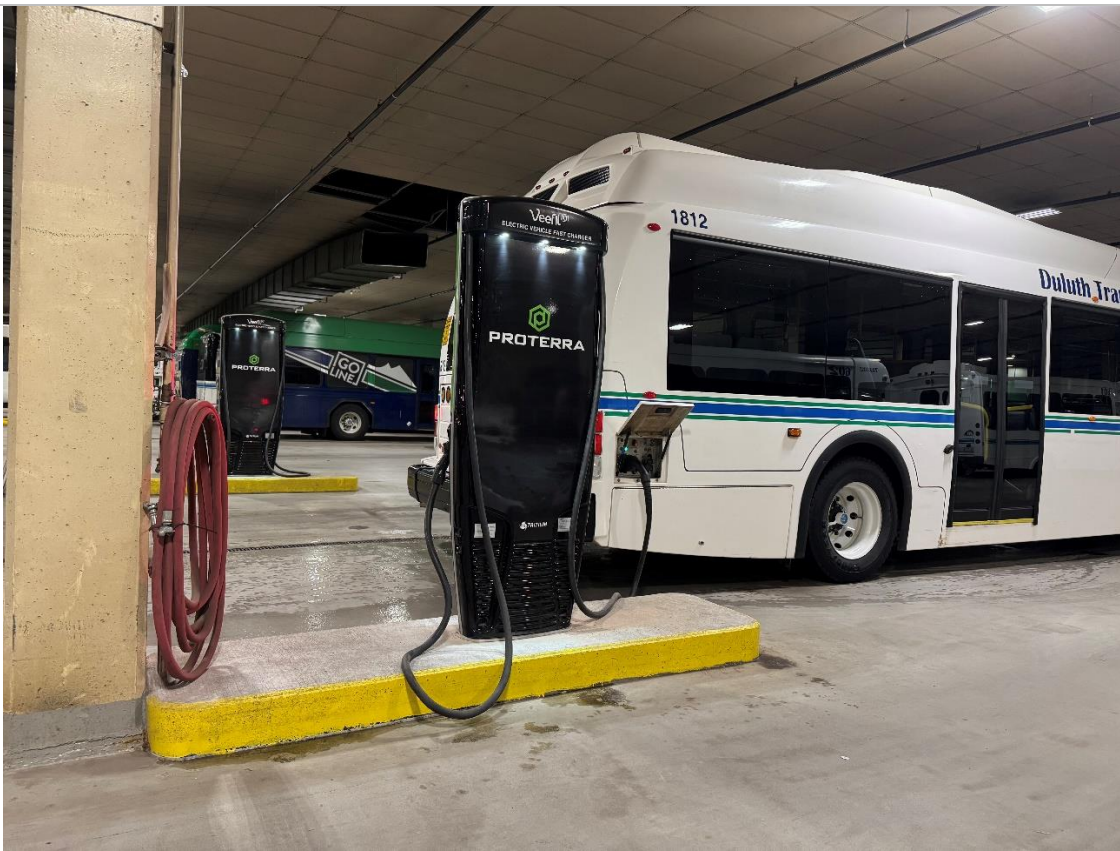
Figure 4 - Side view of Proterra bus receiving a charge from a Tritium RT50 charger. As you can see, charging stations are mounted on concrete pads and connected to charging portals on the right-rear side of the bus. Please note, that concrete pads upon which chargers are mounted, are variable in length; this concrete pad is the shortest of the series of four (4) chargers. 1 ¼" EMT conduit (and ¾" EMT conduit) extend down from the ceiling into the pad, and are routed through the pad to the EVSE. Conduit enters the pad alongside the concrete pillar; near the coiled red hose.
