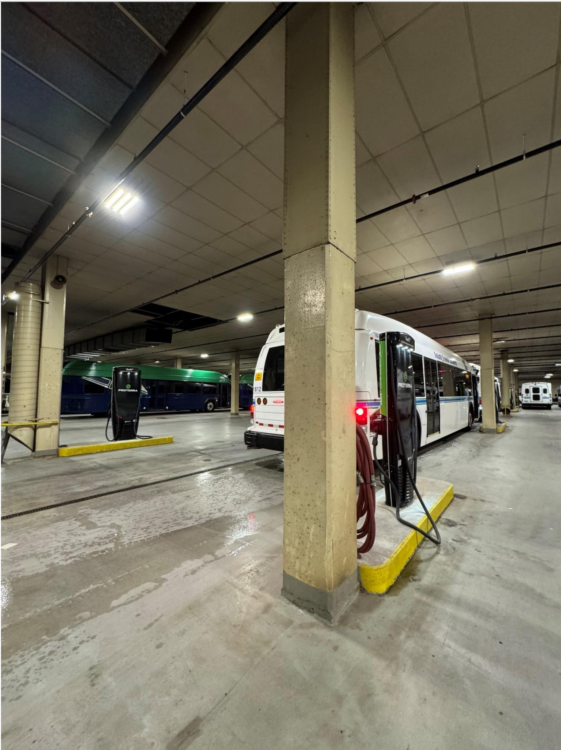
Figure 2 – View of DTA existing EVSE showing that there are two runs of EVSE/charging stations, with a parallel traffic lane between them. A 2017 Proterra Catalyst bus receives a charge from a Tritium RT50 Charger. This example also illustrates the pedestal chargers mounted on concrete pedestals.
