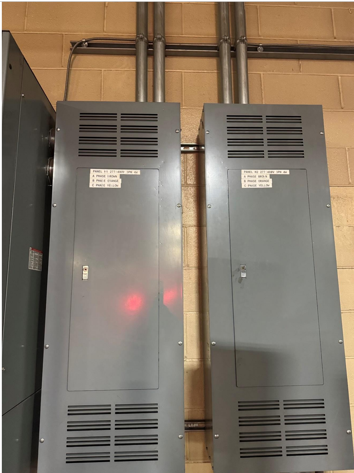
Figure 1- Breaker panels serving DTA's existing charging stations. Each breaker panel is 800 A and circuit breakers are 80A each. Each circuit breaker panel serves a charging "run" consisting of four (4) EVSE/charging stations. Conduit extending from panels into ceiling is 2" EMT.
