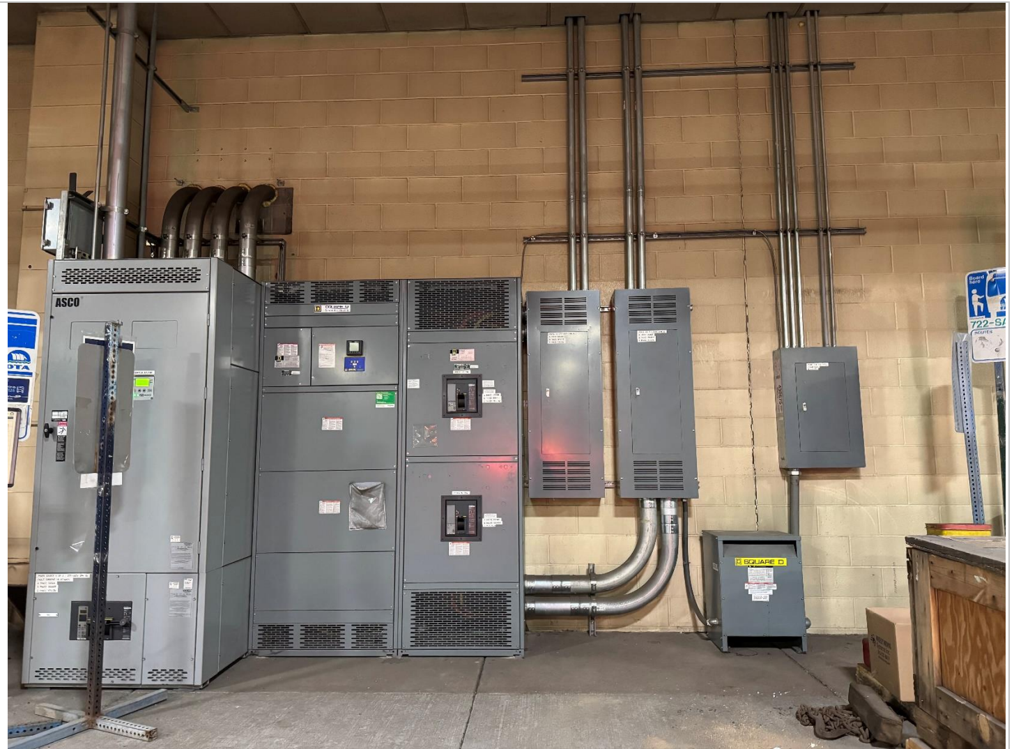
Figure 7 – DTA Electrical Infrastructure. Two sets of 2" conduit extend from circuit breaker panels that serve the DTA's existing eight (8) Tritium RT50 charging stations. Circuit breakers inside the twin breaker panels are 80A each. The DTA does not wish to make modifications to the existing electrical infrastructure upstream of the breakers, and is only willing to upgrade 80 A breakers to 125 A.
