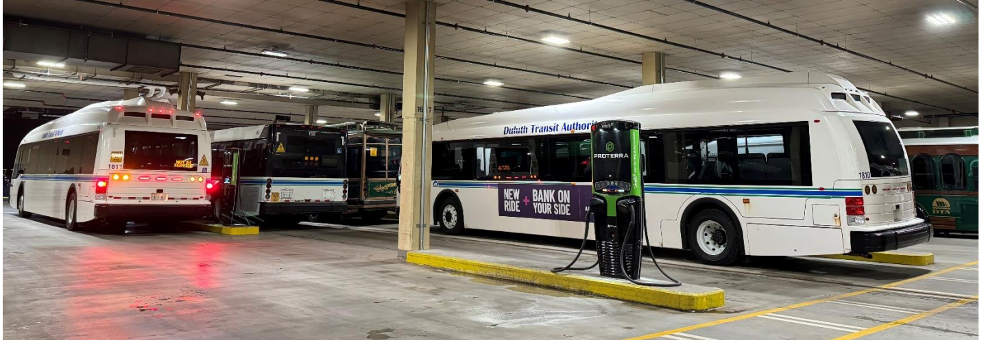
Figure 6 - View of EVSE layout, from near pedestrian walkway (yellow lines on floor). This shows the 3 rd and 4 th chargers in each series of four chargers, with two chargers on each side of the lane on the side of the pedestrian walkway that is hidden from view. Note that these concrete pads are longer, with 1 ¼" EMT drops on the opposite side of the chargers relative to the breaker panel from which the conduit supplying the EVSE originates. Some chargers/concrete pads are hidden from view due to obstructing buses.
