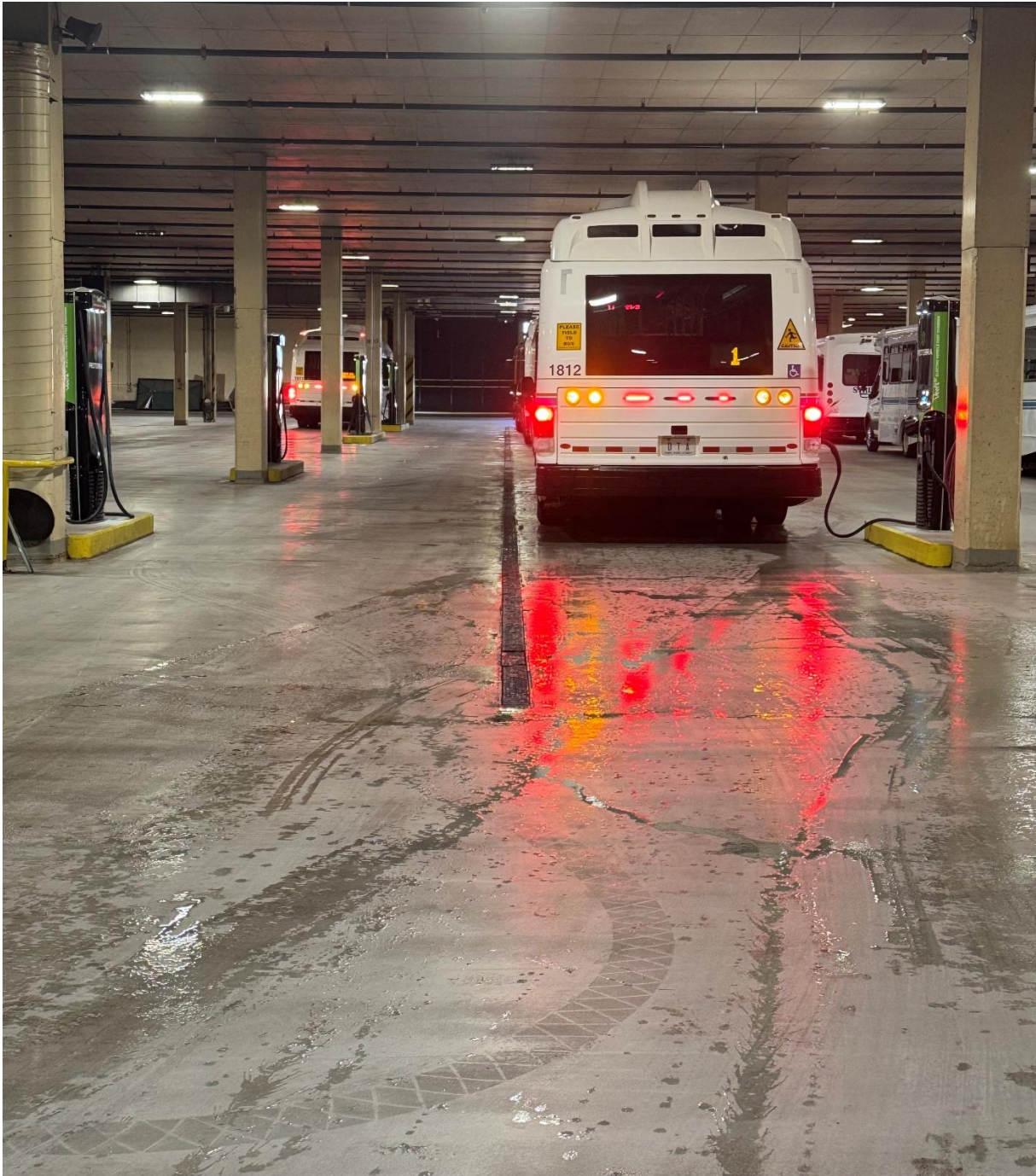
Figure 3- A view from the traffic lane encircling the perimeter of the DTA's bus storage facility taken from the portion of the lane near the breaker panels. Charger layout consists of four (4) EVSE served by each panel, parallel to each other, with EVSE stations mounted on concrete pedestals. A traffic lane to allow the maneuvering of buses alongside the chargers is between each run of chargers. A total of four (4) buses can be parallel parked end-to-end in each run, for a total of eight (8) buses in this area (not all 8 are visible in this image due to obstruction by parked buses).
