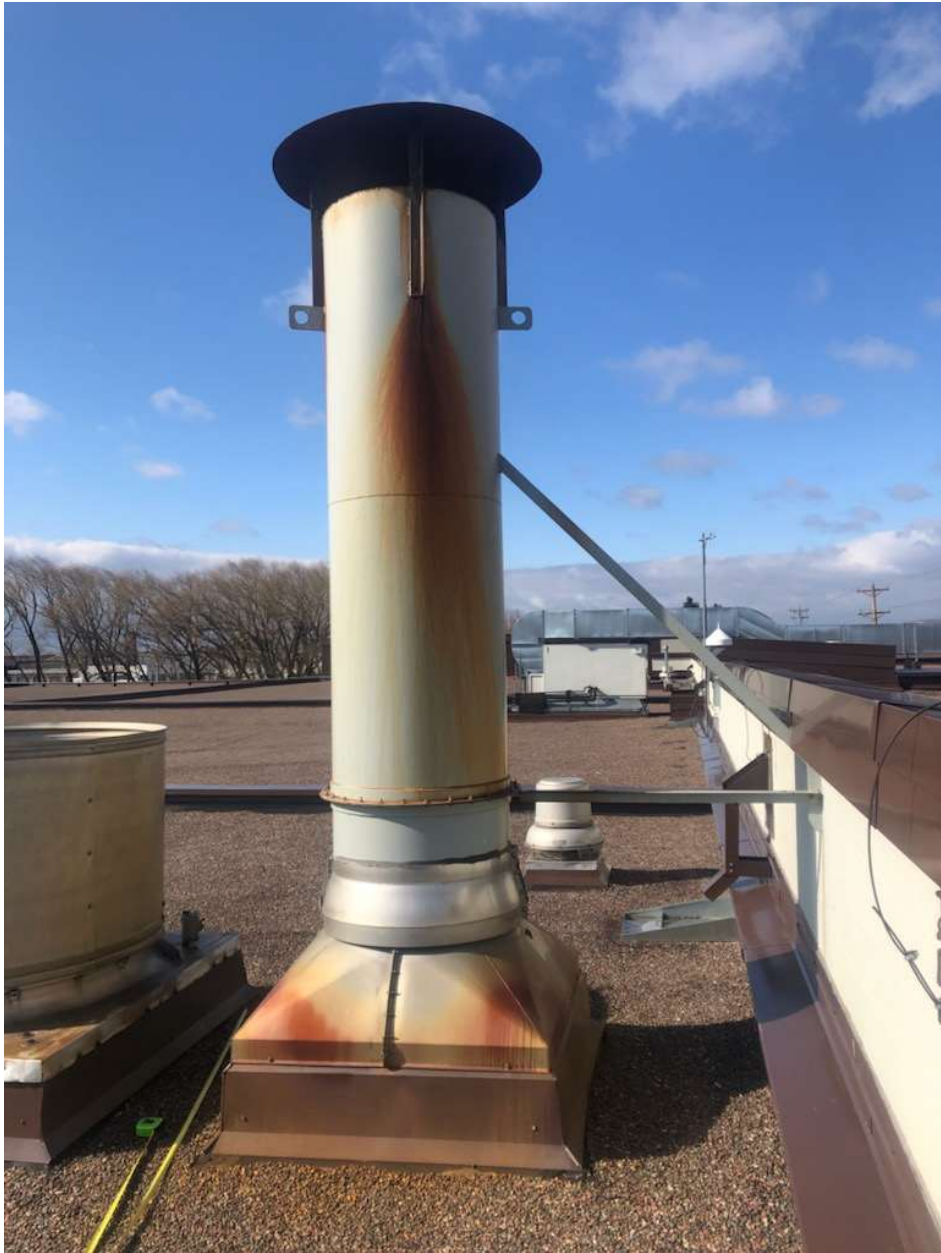
The chimney must also be replaced. The roof was replaced in 2021. It is hot roofing material with a ballast.
