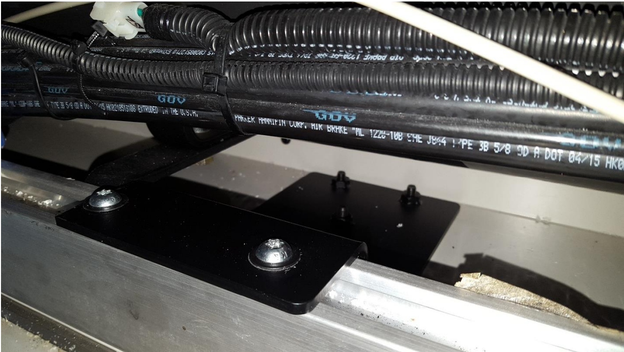
Pictures of the bracket attachment in the electrical cupboard above the driver:
