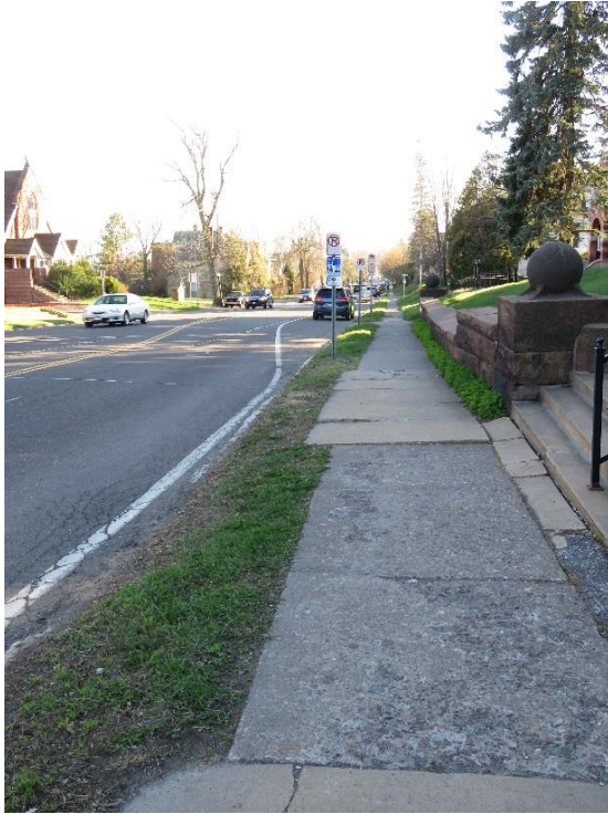
Deteriorated sidewalk adjacent to bus stop
